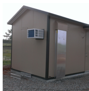
Electric Sub Station
